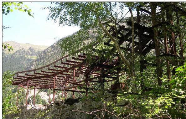
Luisa cableway arrival station
